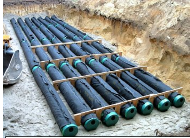
Enviro-Septic ® installed in below ground in a seepage bed drain (leach) field type. Daily Flow Rate is 1,890 litres.
