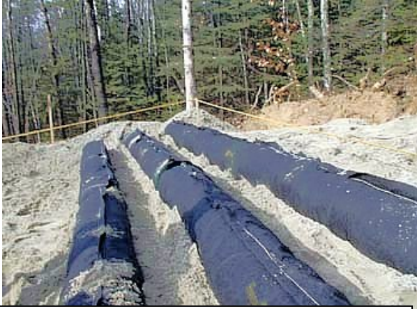
Enviro-Septic ® installed on a slope using a seepage bed drain (leach) field type. Daily Flow Rate is 1,350 litres
