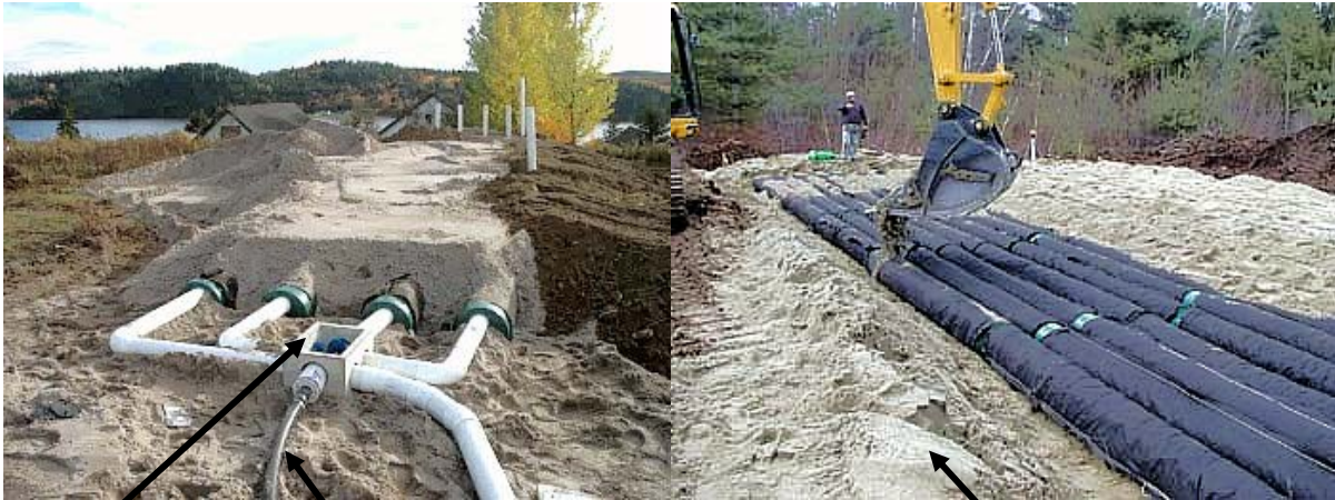
Distribution Box Pump Line from Pre-Tank
